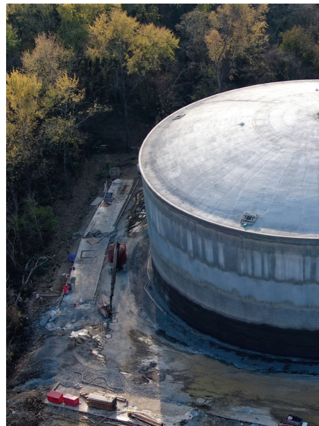
SD1 is adding equalization (EQ) tanks to its system as part of a smart-sewer management program to store excess storm flow and control its release back into our system once a storm is over.
